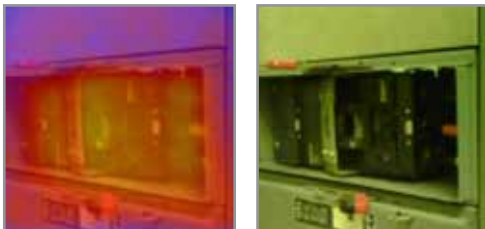
Normal operating temperature on mission critical breaker
